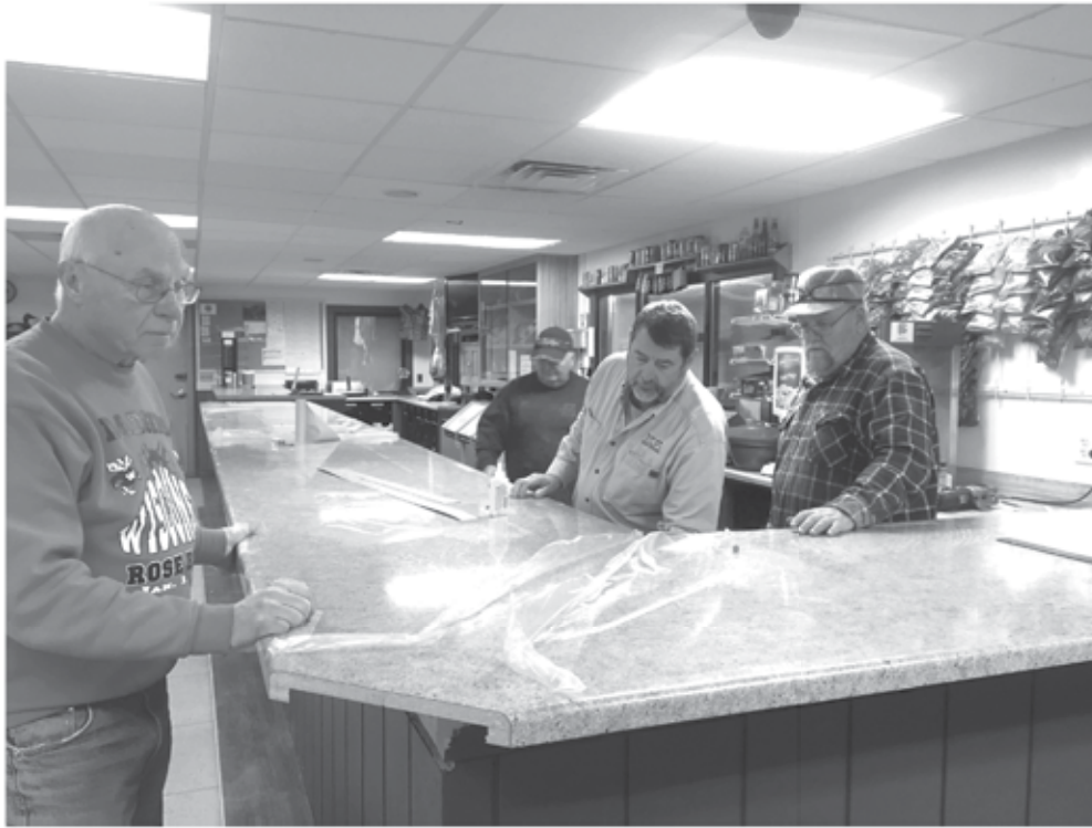
Jerry Reetz, Gene Thom, Steve Beres, & Dave Polzin install the new bar top in the club house.
